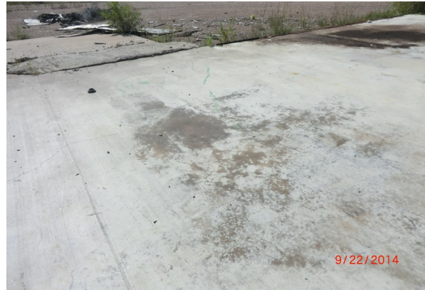
PHOTOGRAPH NO. 6 View staining on concrete pad looking south
