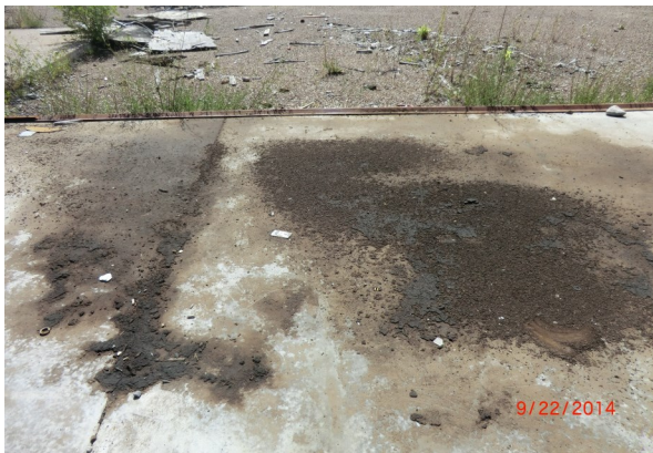
PHOTOGRAPH NO. 7 View staining on concrete pad looking south
