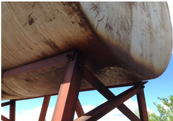
PHOTOGRAPH No. 24 View of corrosion on tank
