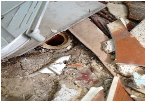
PHOTOGRAPH NO. 28 View of sewer connection in restroom of break room building
